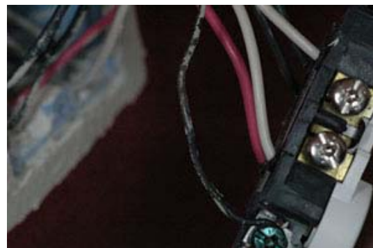
Black corrosion on wiring
