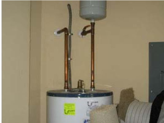
Normal copper plumbing
