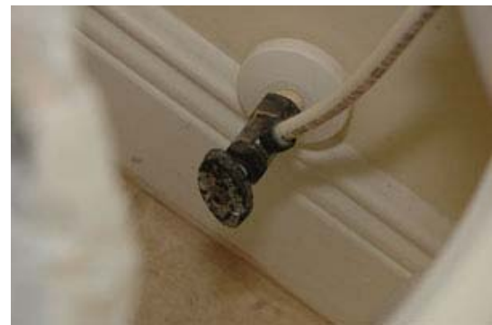
Corroded shut off valve
